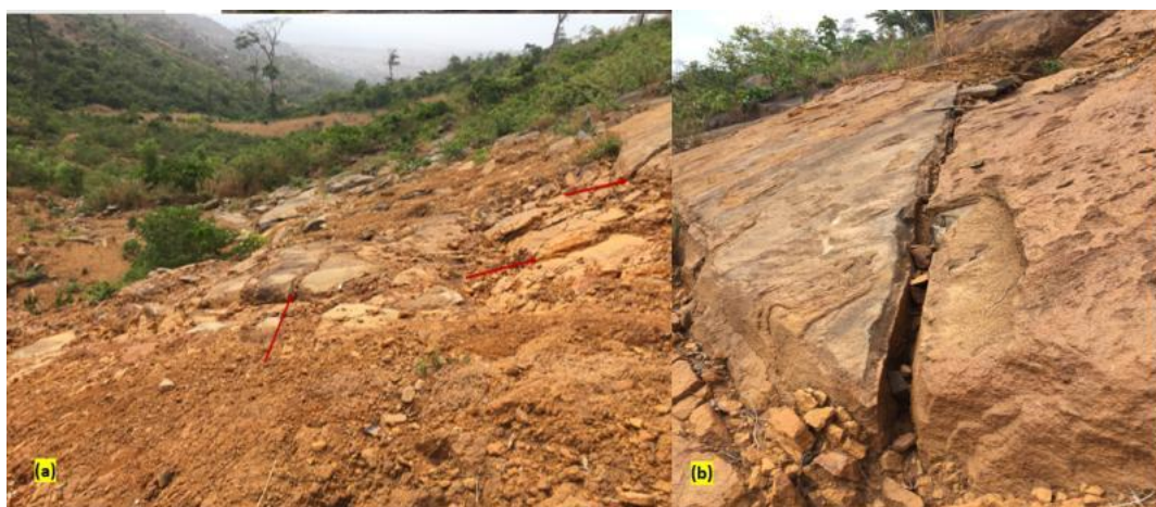
Figure 5. (a) Joint Sets (Vertical Dip) in Highly Weathered Pegmatitic Gabbro, (b) The Largest Offset Fracture (15mm) within the Landslide Area
