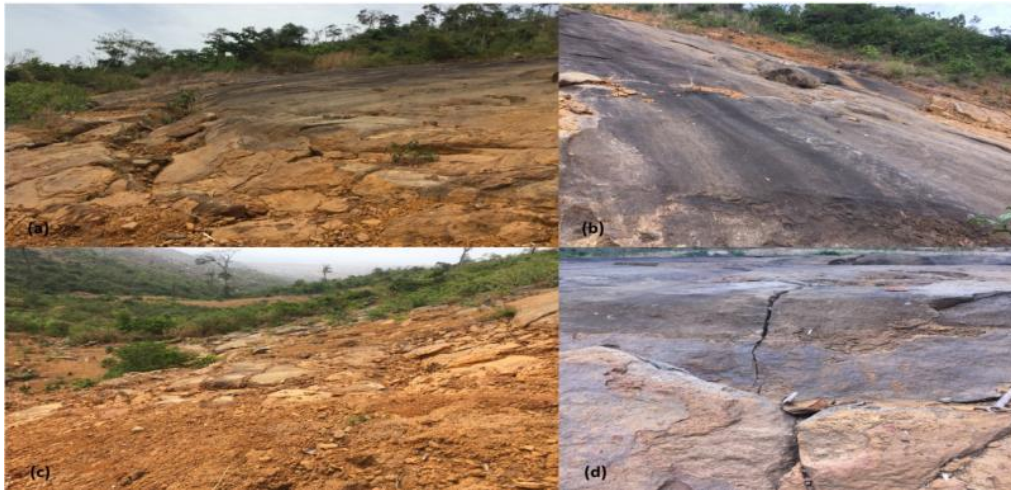
Figure 4. Local Geology (a) Distinct Zones along Slope Face Showing Differential Weathering, Separated by a Transverse Crack, (b) Typical Rock Type with Evidence of Exfoliation Joints, (c) Intensely Weathered Landslide Basal Section Where the Slippage/Failure may Have Initiated, (d) Parallel Proto-Joints in the Process of Developing as Full Mechanical Fractures but Maintaining Considerable True Cohesion
