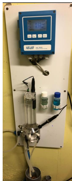
Figure 7. Current Chlorine Meter
