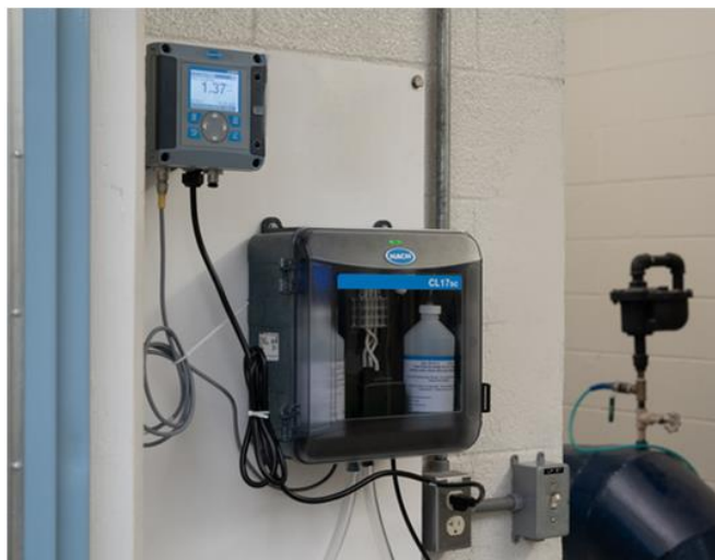
Figure 8. New Chlorine Meter
