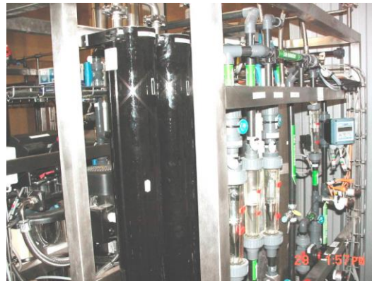
Figure 1. Reverse Osmosis System (Black Cylinders)
