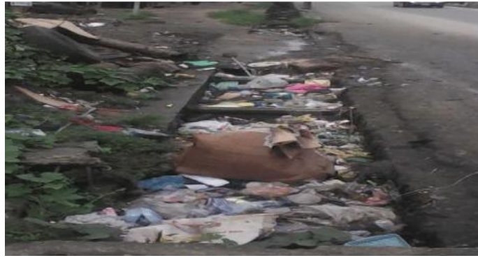
Plate 4. Blockage of Drainage with Solid Waste
