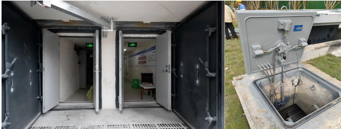
Figure 7. Protective Equipment for Entrances, Exits, and Emergency Exits in Underground Utility Tunnels
