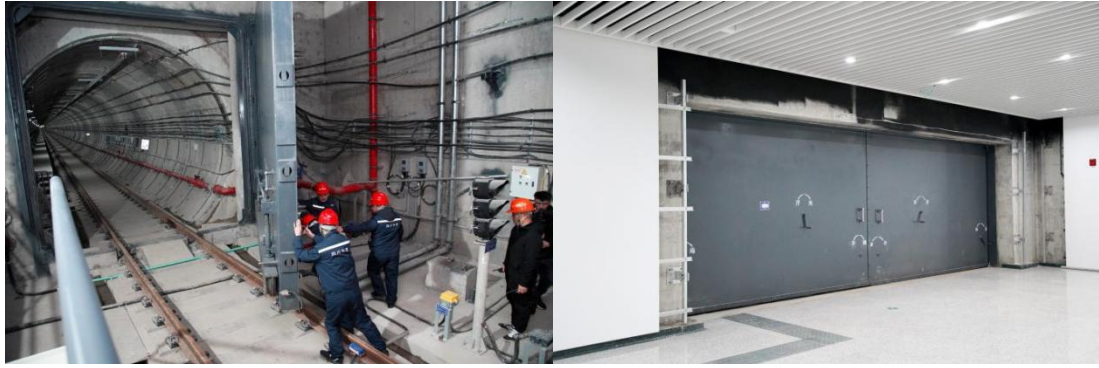
Figure 6. Protective Equipment for Track Areas and Wartime Entrances and Exits at Subway Stations
