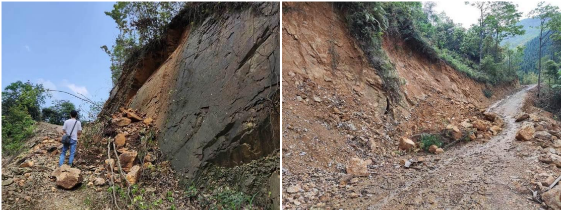
Figure 1. Field Photographs of Collapse B1 and B2
