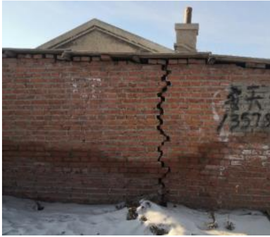
Figure 3. Cracks in the Exterior Wall of the House
