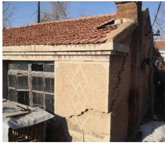
Figure 6. Cracks at the Top of the Exterior Wall of the House
