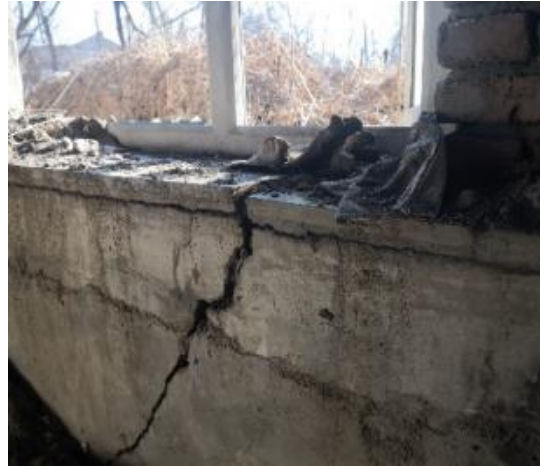
Figure 4. Cracks in the Perimeter Wall
